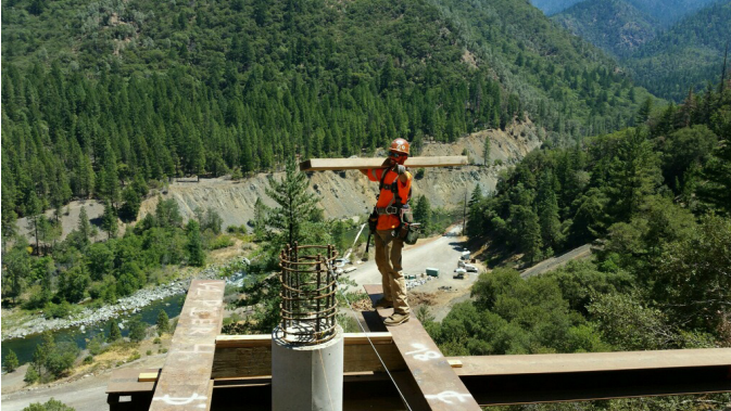
Workers faced severe fall hazards on the Collins Curve project.
